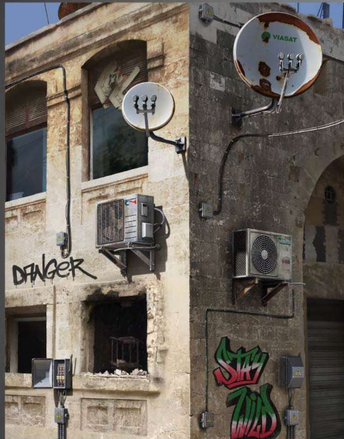
35638 AIR CONDITIONERS & SATELLITE DISHES
